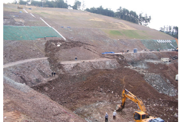
Fig. 2. slope failure in cut slope of rail road
